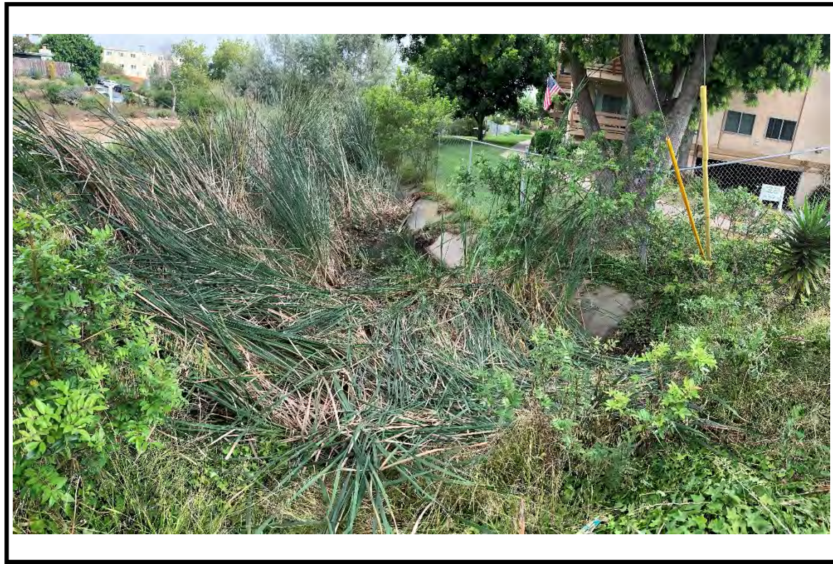
Photo Point 6. View of concrete lined channel that drains the urban watershed into Pond 1. Channel choked with sediment and vegetation. Photo date: 8/24/23. Direction: north.
