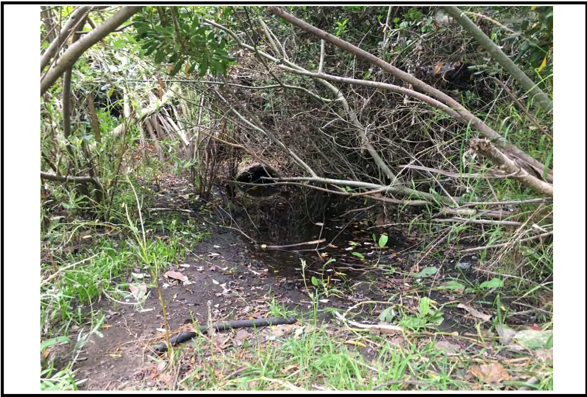
Photo Point 1. View of sediment filled culvert inlet in Pond 1. Photo date: 8/8/23. Direction: south.
