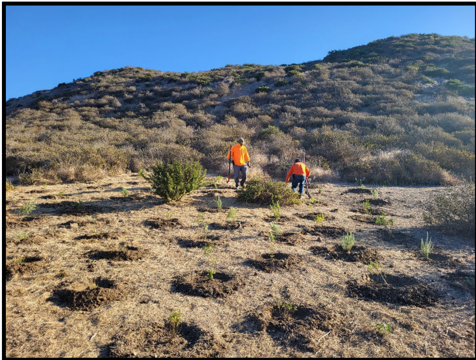
On 11/3/23, Habitat West installed native plants in the SW and NE project areas.
